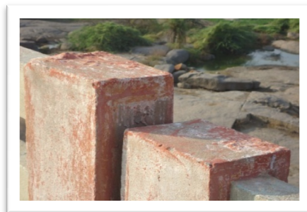
Figure 3: Level Difference Observed in Hand Rail at Pier P-11 & Pier P14
