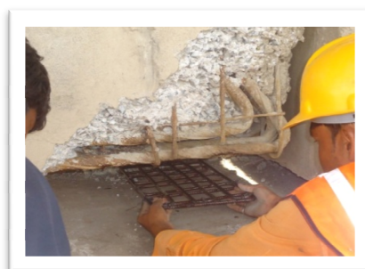
Figure 4: Reinforcement Bars Exposed At the Bearing Region of Main Girder
